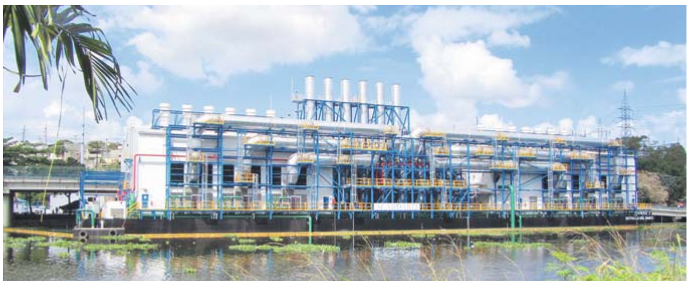
■ Fig. 14 – A moored power barge.
