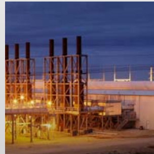
Flexible grid stability power plants
