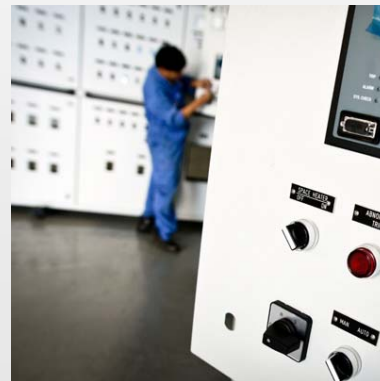
Electrical & automation services
