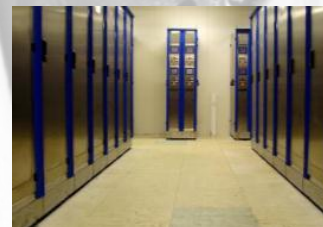
Power electric systems
